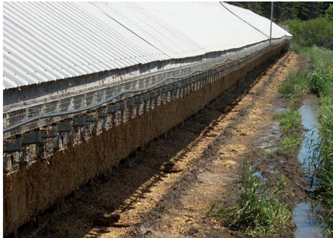
Poor drainage around shed which creates ideal fly breeding area.
