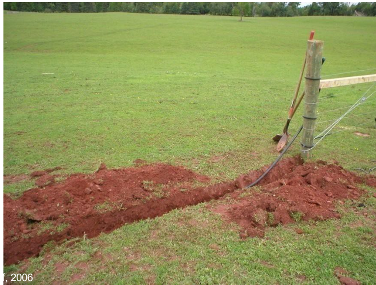
Figure 3.6 Wire runs through a water hose underneath a gate.
