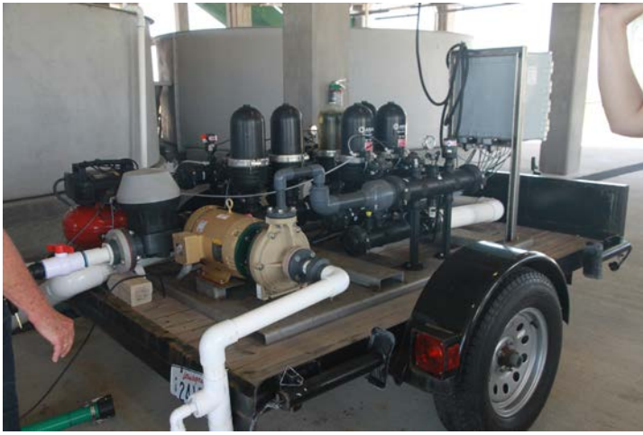
FIGURE 1. Filtration equipment installed on a trailer with quick disconnect and union fittings at the Louisiana Sea Grant Oyster Research Hatchery in Grand Isle, Louisiana. Photo courtesy of University of Florida/IFAS Shellfish Extension
