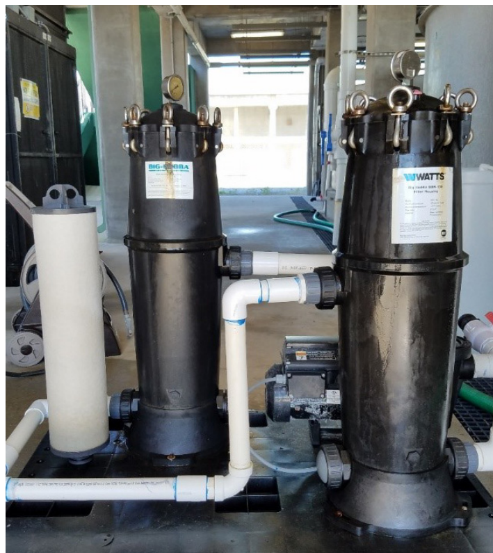
FIGURE 2. Filtration equipment installed on a pallet with quick disconnect and union fittings at the Louisiana Sea Grant Oyster Research Hatchery in Grand Isle, Louisiana. Photo courtesy of John Supan
